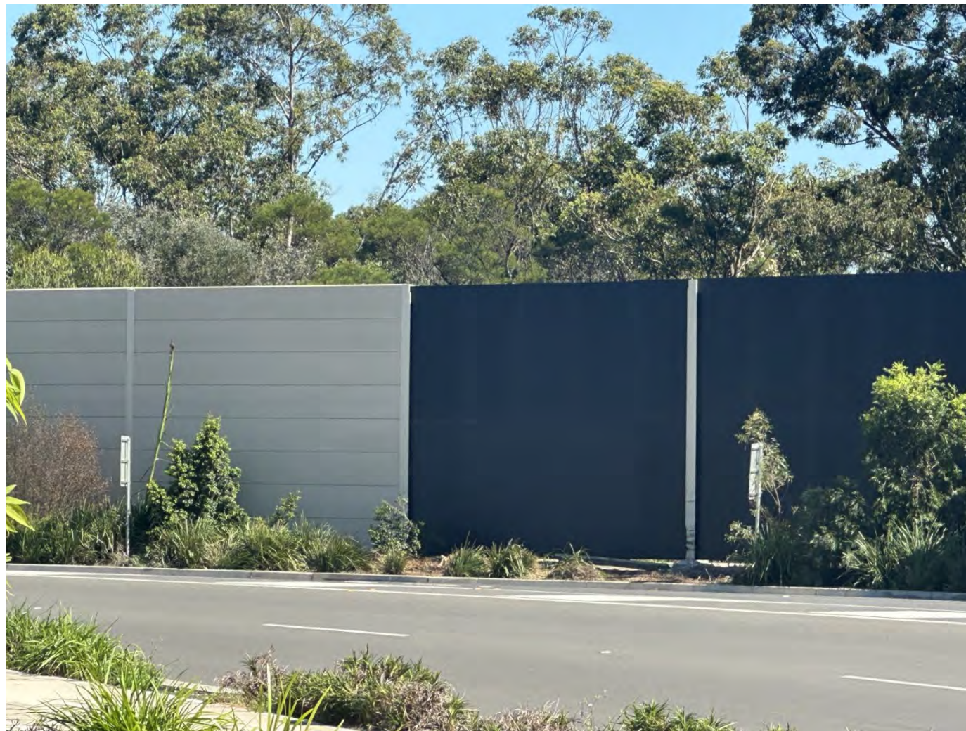
Figure 47 - Mortality amongst noise wall ground cover vegetation (09/04/2026)
