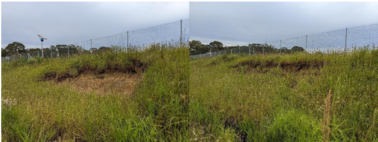
Plate 9. Batter slumping observed within the Rail Link
