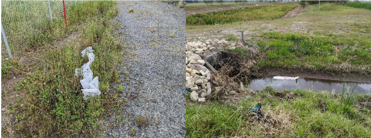
Plate 8. Litter observed within the rail corridor and IMEX, warehouses and drainage infrastructure during the October inspection
