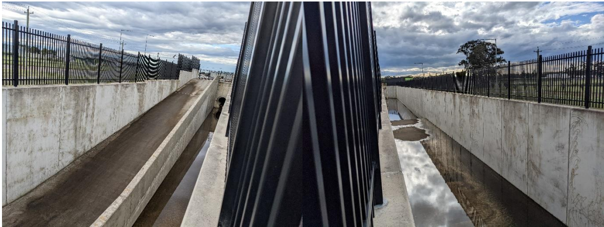
Plate 4 Northern drainage area of MPE with lack of any plant growth
