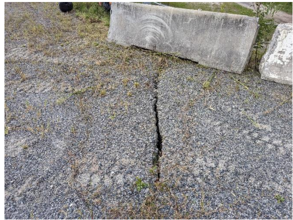
Plate 9 Batter slumping observed within the Rail Link (left) and concrete platform cracking (right)
