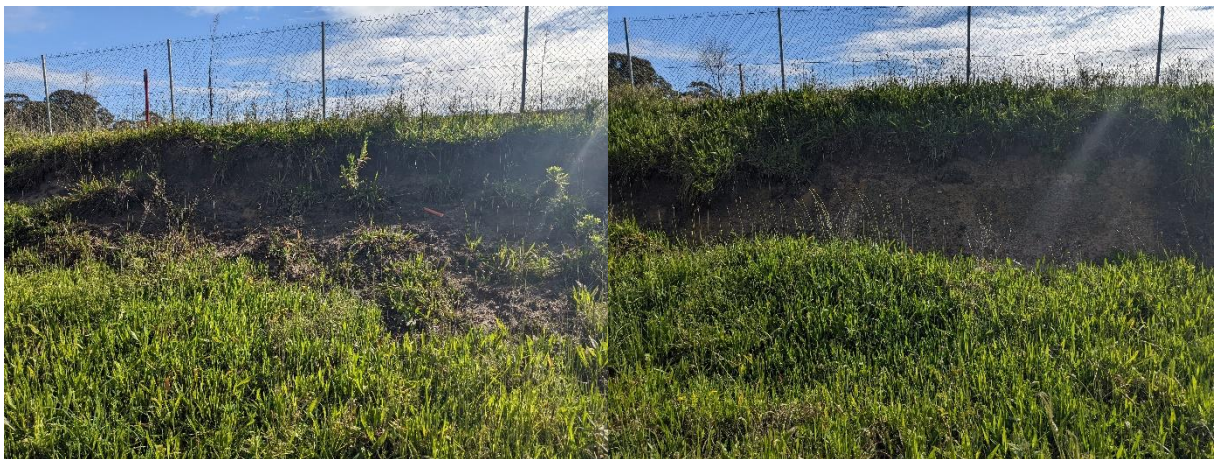
Plate 9. Batter slumping observed within the Rail Link
