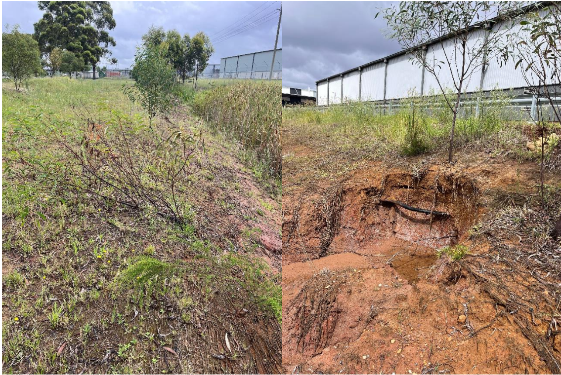
Plate 2. Observation of native plant damage and erosion in drainage basins.
