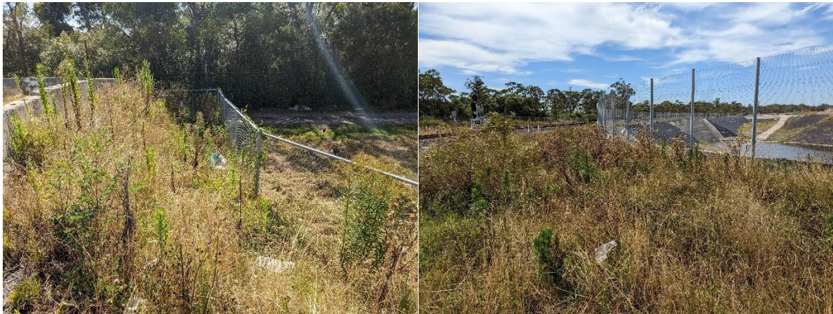
Plate 8. Exotic species continue colonising remediated soft batters within the Rail Link corridor
