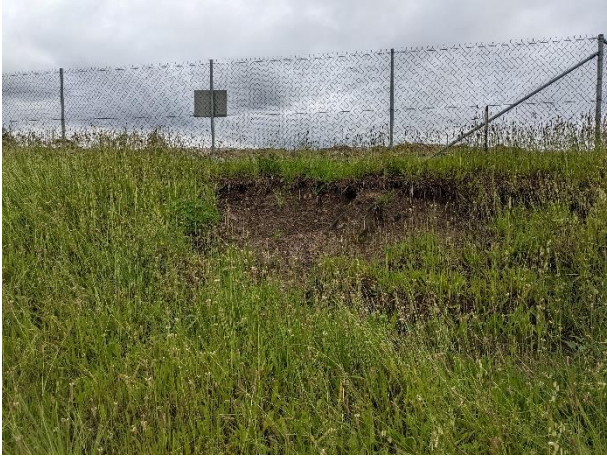
Plate 10 Batter slumping observed within the Rail Link
