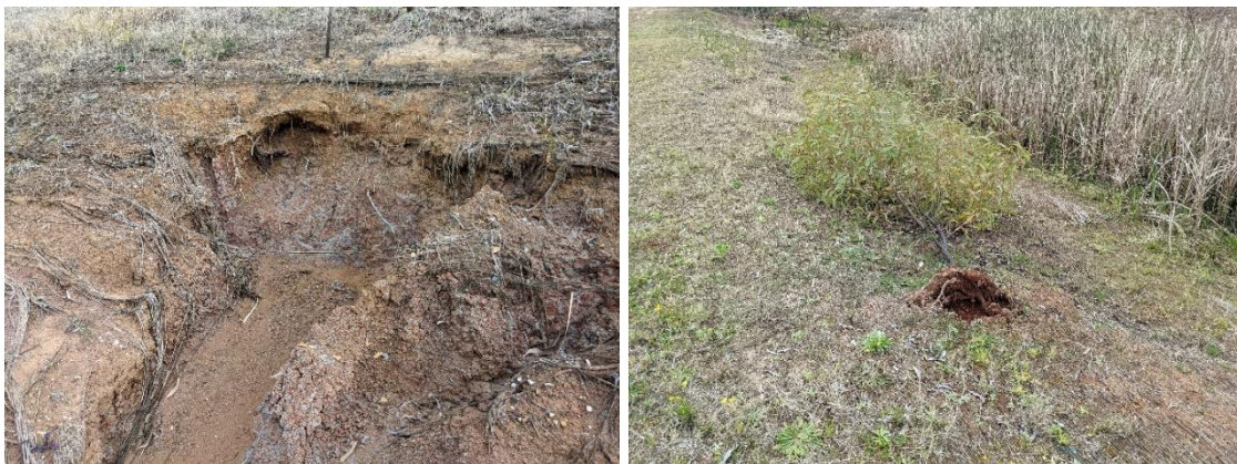
Plate 2. Observation of native plant damage and erosion in drainage basins. Observations were also present in the July 2022 survey.
