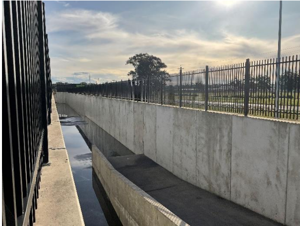
Plate 3 Northern drainage area of MPE with lack of any plant growth
