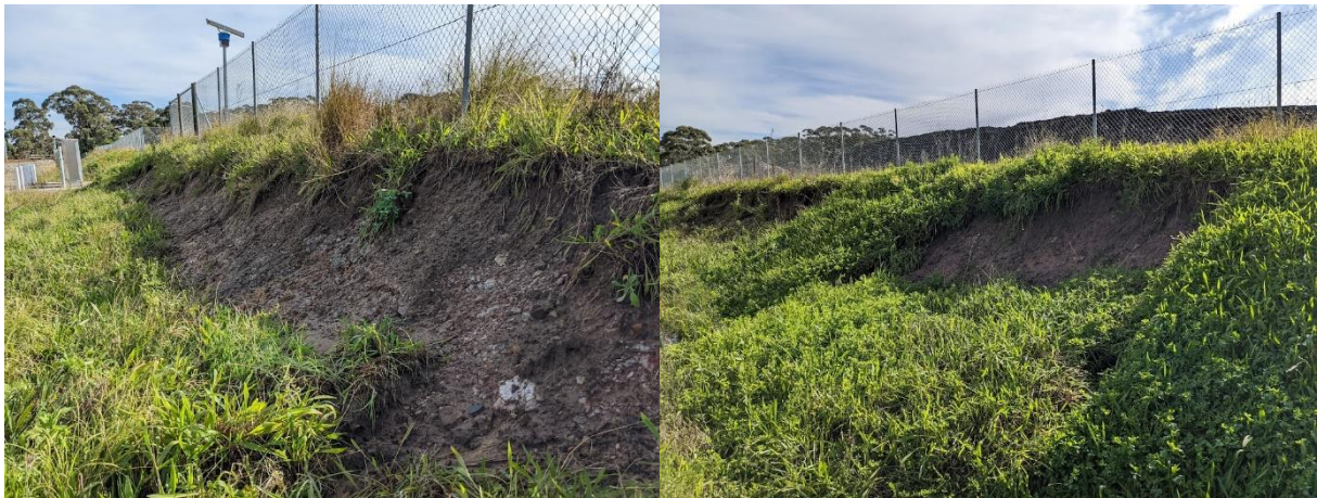
Plate 8. Batter slumping observed within the Rail Link
