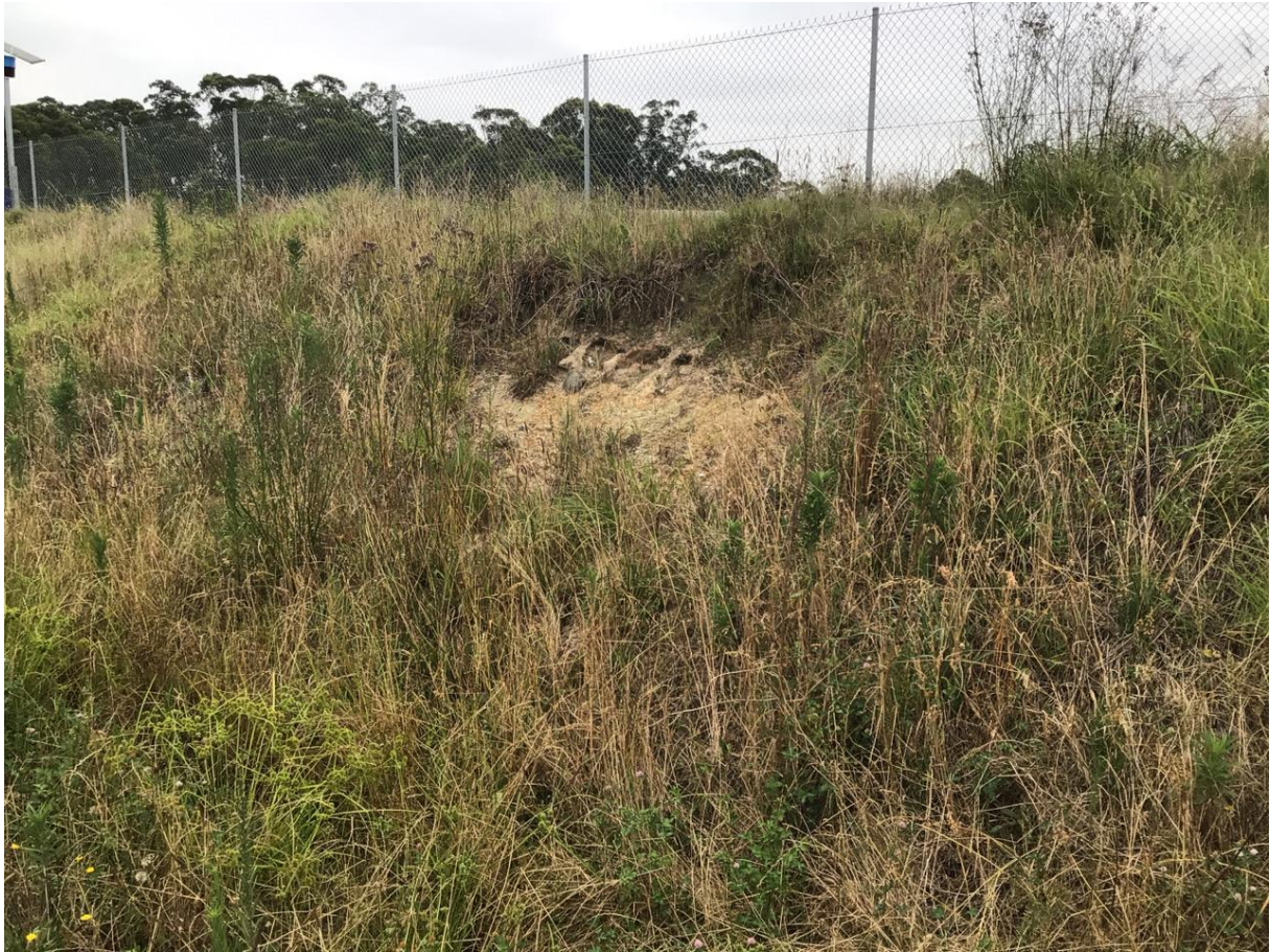
Plate 5. A section of soft batter which has slumped within the Rail Link
