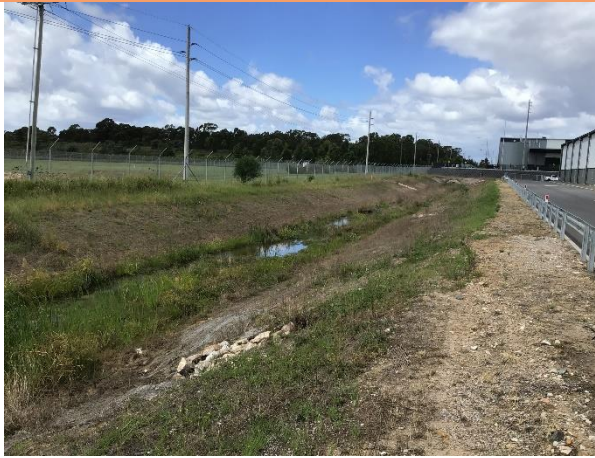
Weeds beginning to colonise drainage swales and basins at the north-eastern extent of facility
