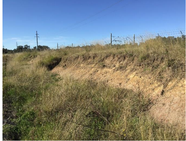
Slumping of soft batter within the Rail Link.
