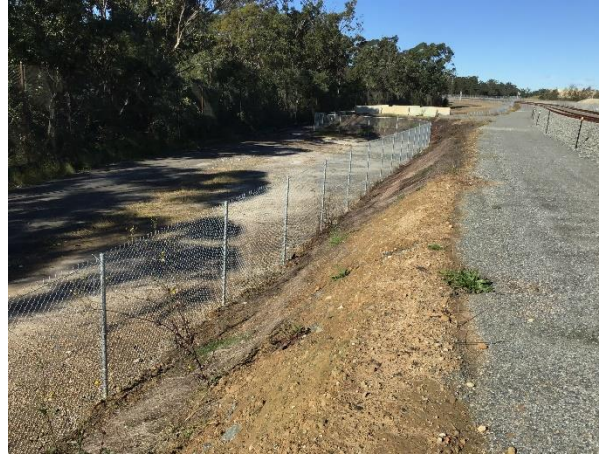
Exposed soft batters that are susceptible to weed invasion along the Rail Link.
