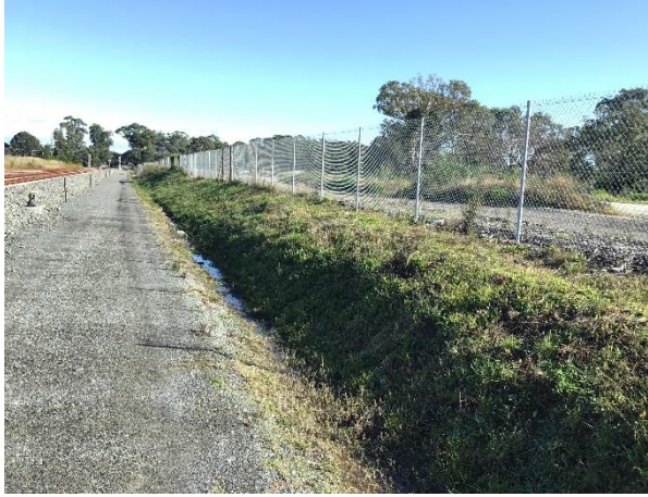
Slashing of exotic grasses observed along the rail corridor.
