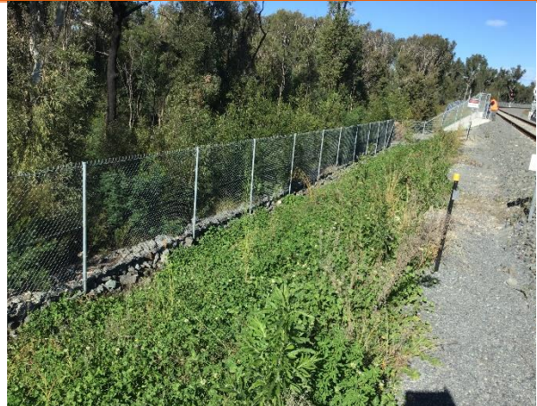
Batter dominated by White Clover that should be cut back from the Rail Link fence to avoid encroachment in adjacent native bushland.
