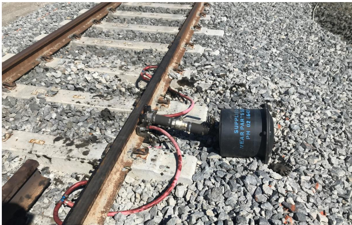
Figure 2 Existing friction modifier installed on Curve 1
