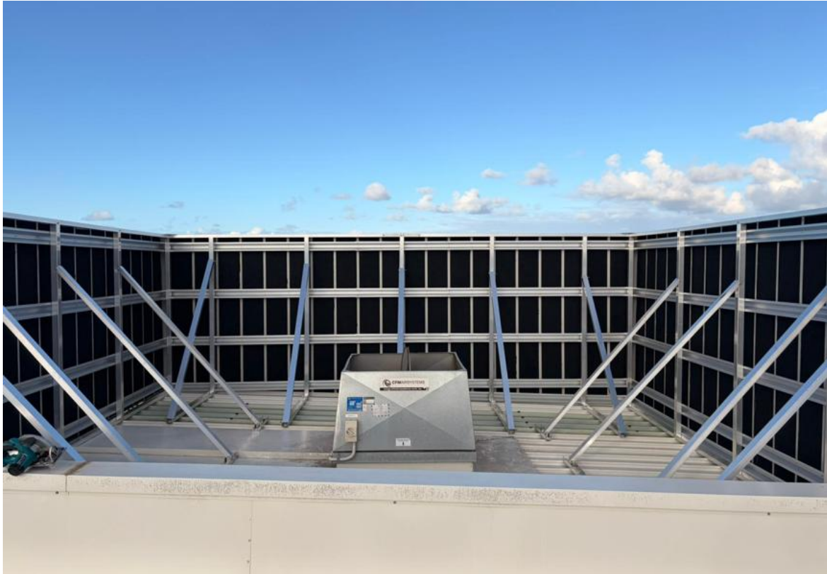
Figure 1: Acoustic screen at Warehouse E7
