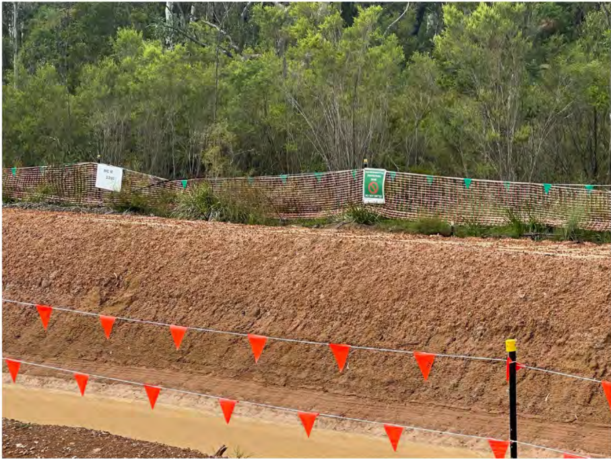
Photo 16: Sediment basin and no go advisory signage
