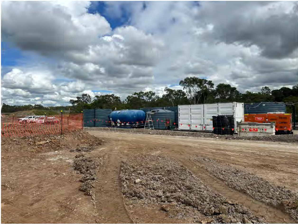
Photo 5: Water treatment plant
