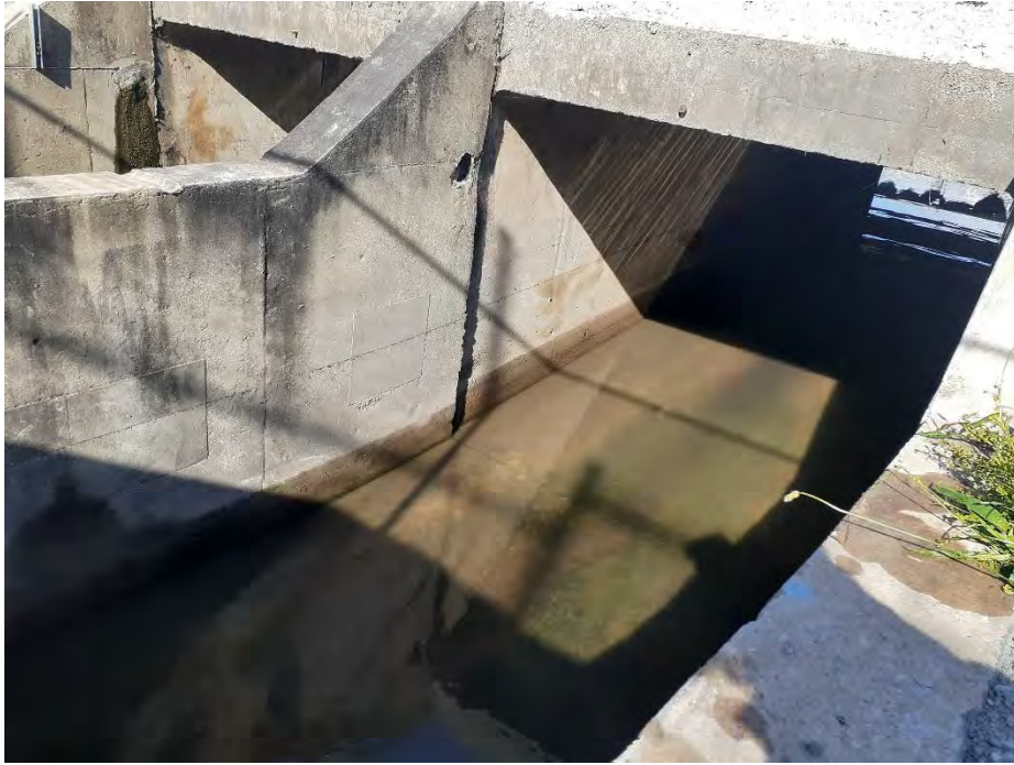
DP-2 STORMWATER CULVERT (POOL 0.5M DEPTH) TO THE NORTH WEST OF THE (EAST PRECINCT)
