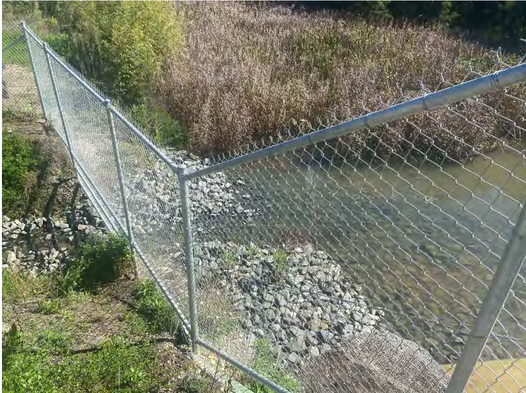
DP-5 FLOWING WATER AT RAILWAY BRIDGE CULVERT ANZAC CREEK
