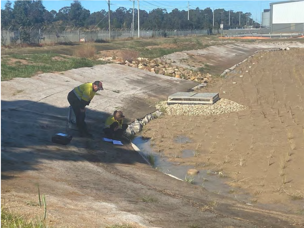
DP-1A) (DETENTION POND) MONITORING TEST SITE (TESTING SHALLOW POOLS – RESIDUAL STORAGE POST RAINFALL EVENT (2 DAYS AFTER)
