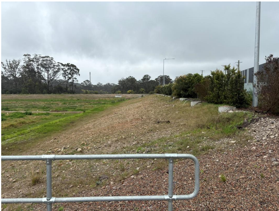
OSD 6 showing batters without topsoil or vegetation.
