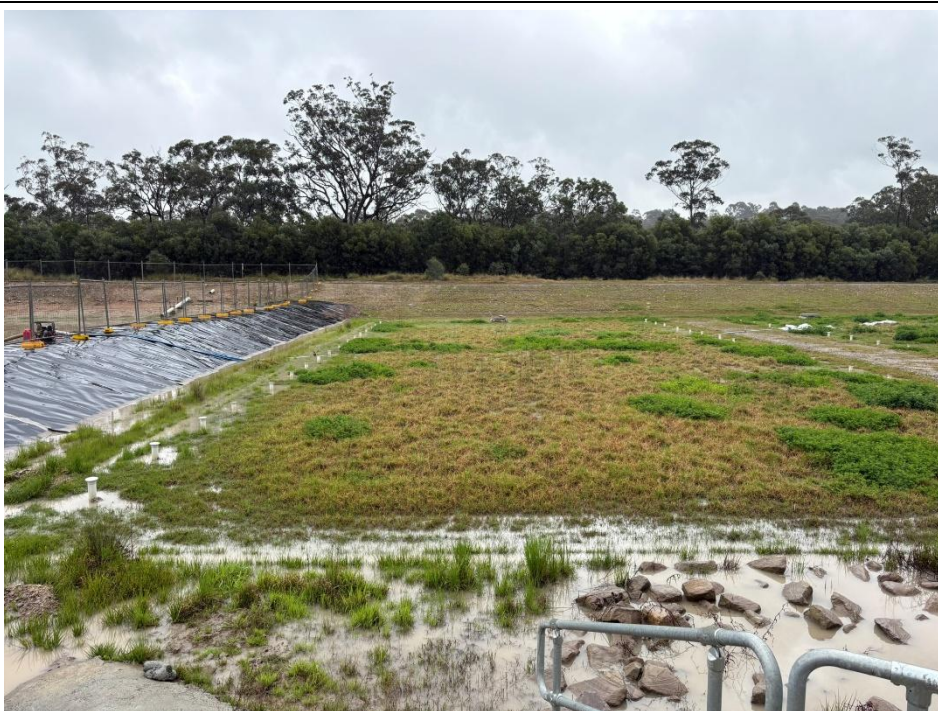
OSD 8 Sacrificial state with HDPE lined batters and pump out operation from the adjacent sediment basin into the biocells. This basin also perimeter mowing with an appearance of diminished flow directed to centre of basin.
