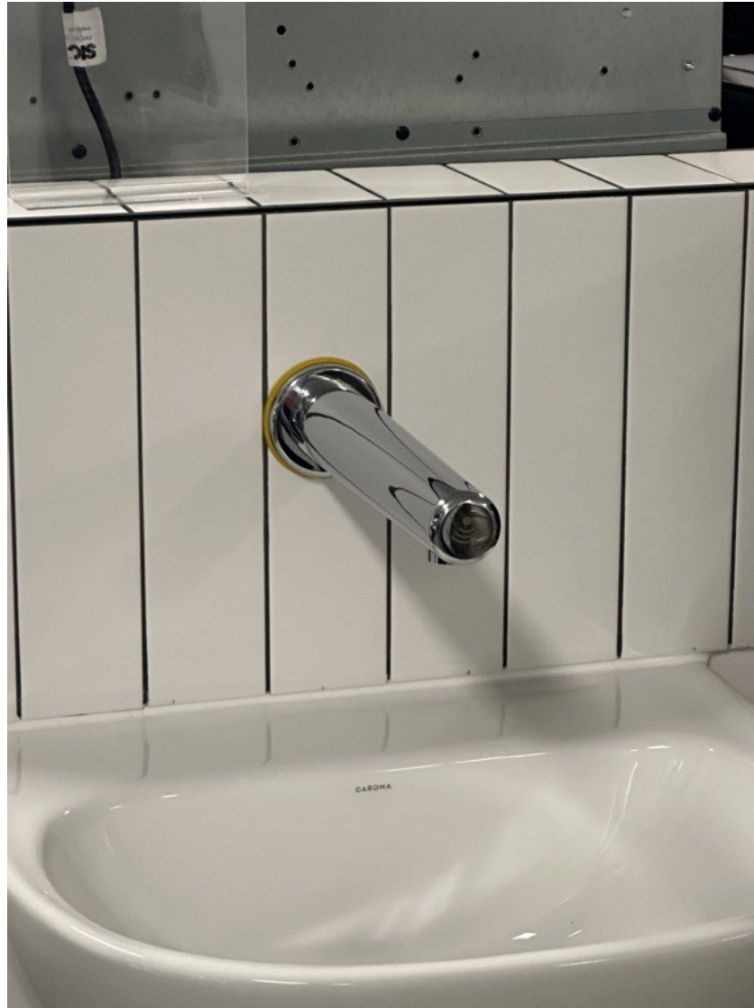
Figure B49 - 17 Water efficient tap at warehouse N1
