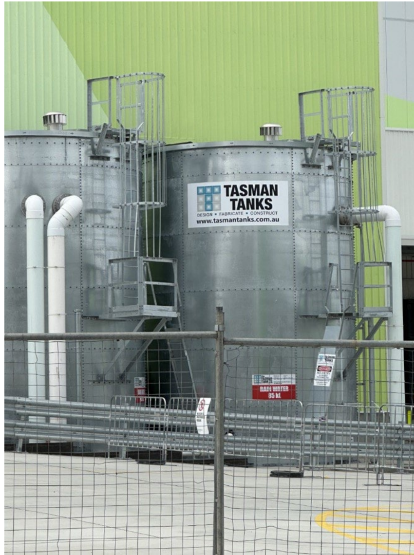
Figure B48 - 7 Operational rainwater tank at warehouse JR
