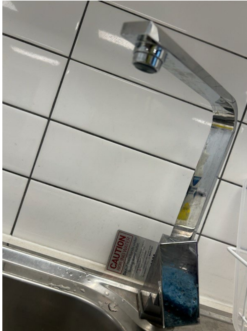
Figure B49 - 16 Water efficient tap at warehouse N2
