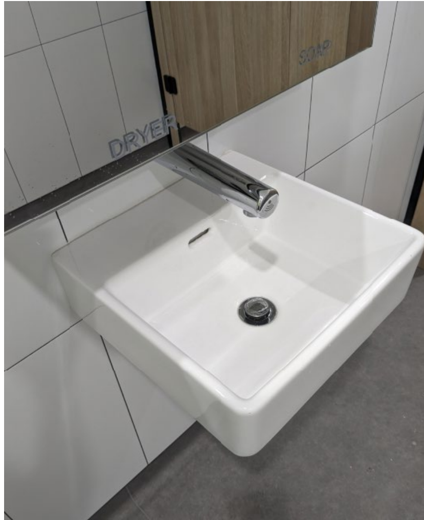
Figure B49 - 15 Water efficient tap at warehouse JR
