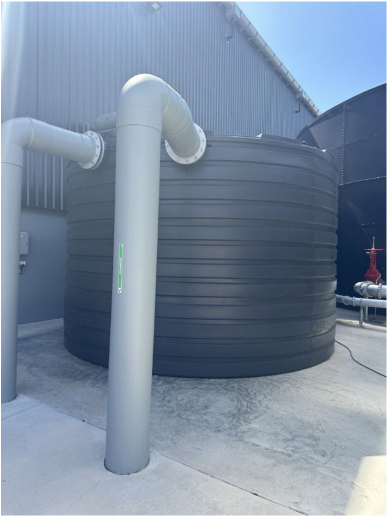
Figure B48-6 – Operational rainwater tank at warehouse N1
