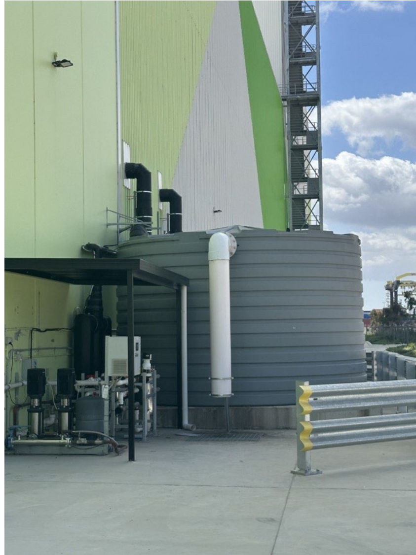
Figure B48 - 8 Operational rainwater tank at warehouse JN
