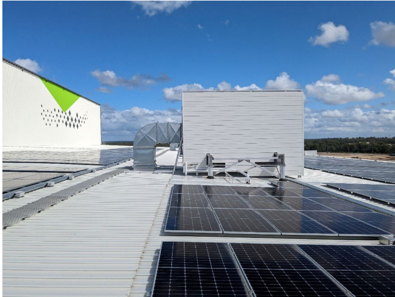
Figure B48 - 14 Roof of warehouse JN with low albedo material installed
