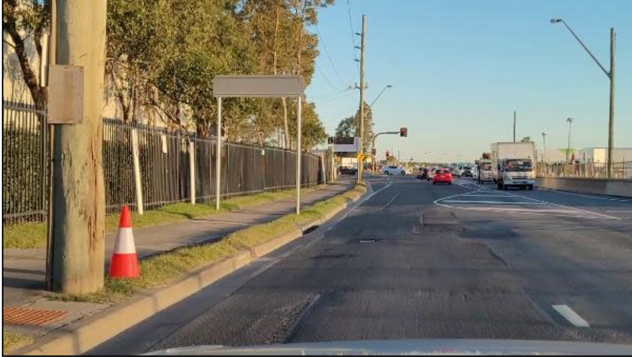
PHOTO 7: For travel along Moorebank Avenue at the Bapaume Road intersection, there are sections of poor pavement resulting in sub-standard ride quality and delineation.
