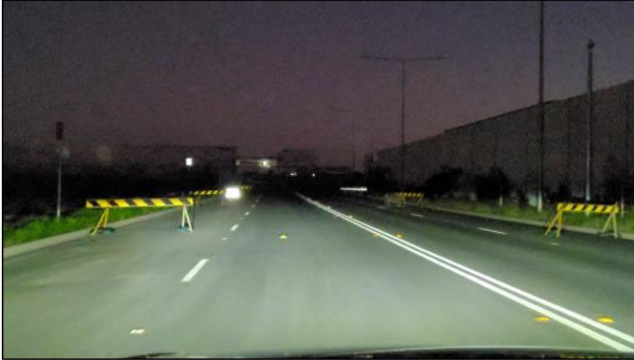
PHOTO 3: For travel along the Western Ring Road, the street lighting was not operational resulting in a darker section of road network in comparison with adjacent road sections.
