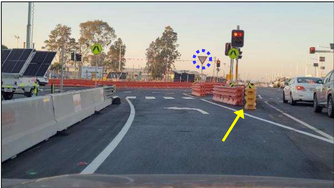
PHOTO 10: For the approach to the Anzac Road left-turn splitter island for Moorebank Avenue southbound travel, the temporary safety barrier ends do not have hazard markers to adequately delineate them. Also, note the 'Give Way' sign located on the right side of the approach only, which is non-standard and should be duplicated on the left side to reinforce the intersection control
