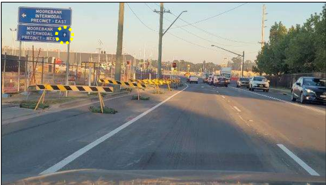
PHOTO 12: For Anzac Road westbound travel, the directional sign for 'Moorebank Intermodal – West / ABB Australia' has an arrow that appears to be too small in size and is inconsistent with the arrow size for the adjacent 'Moorebank Intermodal – East' sign.
