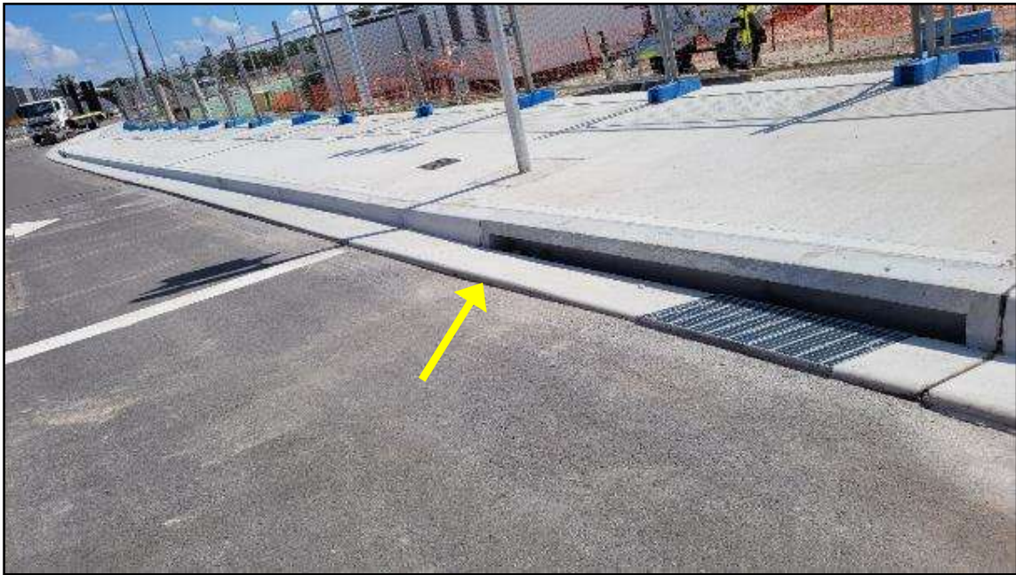
PHOTO 11: On Bushmaster Avenue, there is a lip between the temporary, incomplete pavement surface and the gutter and drains. This may result in excessive water ponding and extending into the adjacent travel lanes.
