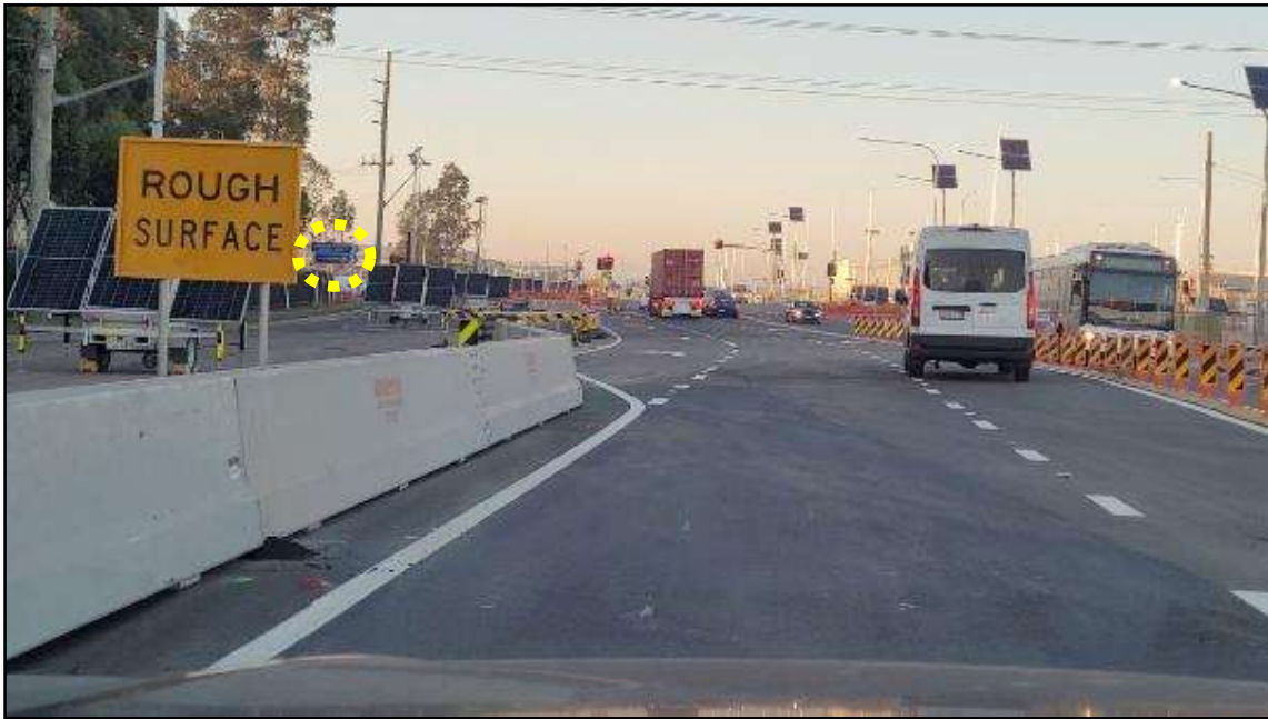
PHOTO 5: For Moorebank Avenue southbound travel, the intersection direction signage approaching Bushmaster Avenue is located too far to the left of the approach travel path and is obstructed by lighting solar panels and other work-site obstructions. Moreover, the signage would be better located to the right to reflect the destinations it is directing to.
