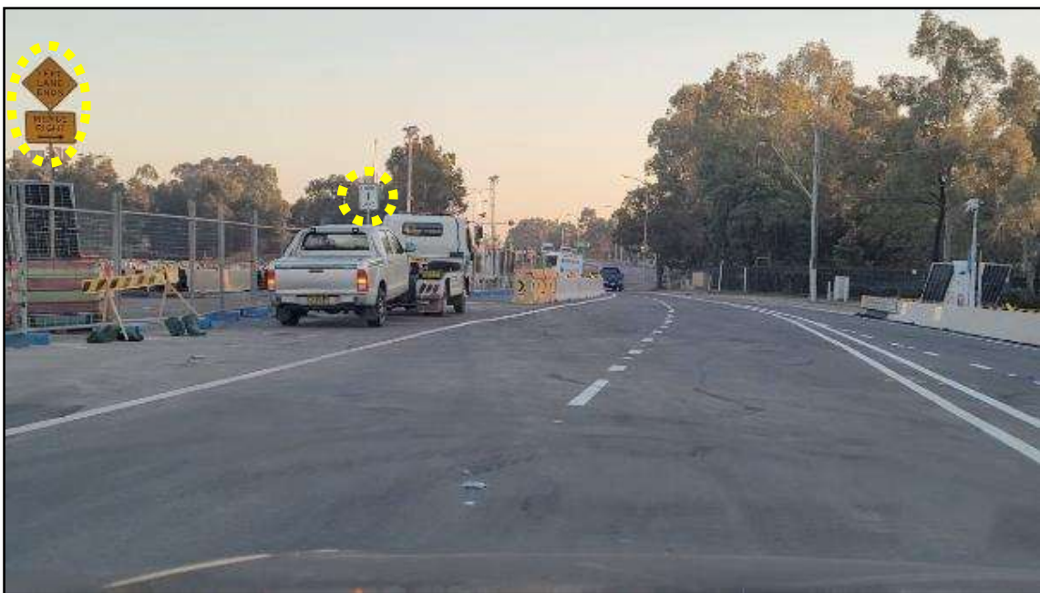
PHOTO 4: For Moorebank Avenue northbound travel, the lane-drop north of Bapaume Road is poorly defined with a lack of merge arrows and the 'Left Lane Ends / Merge Right' and 'Form 1 Lane' signage being located too far left of the approach travel path.
