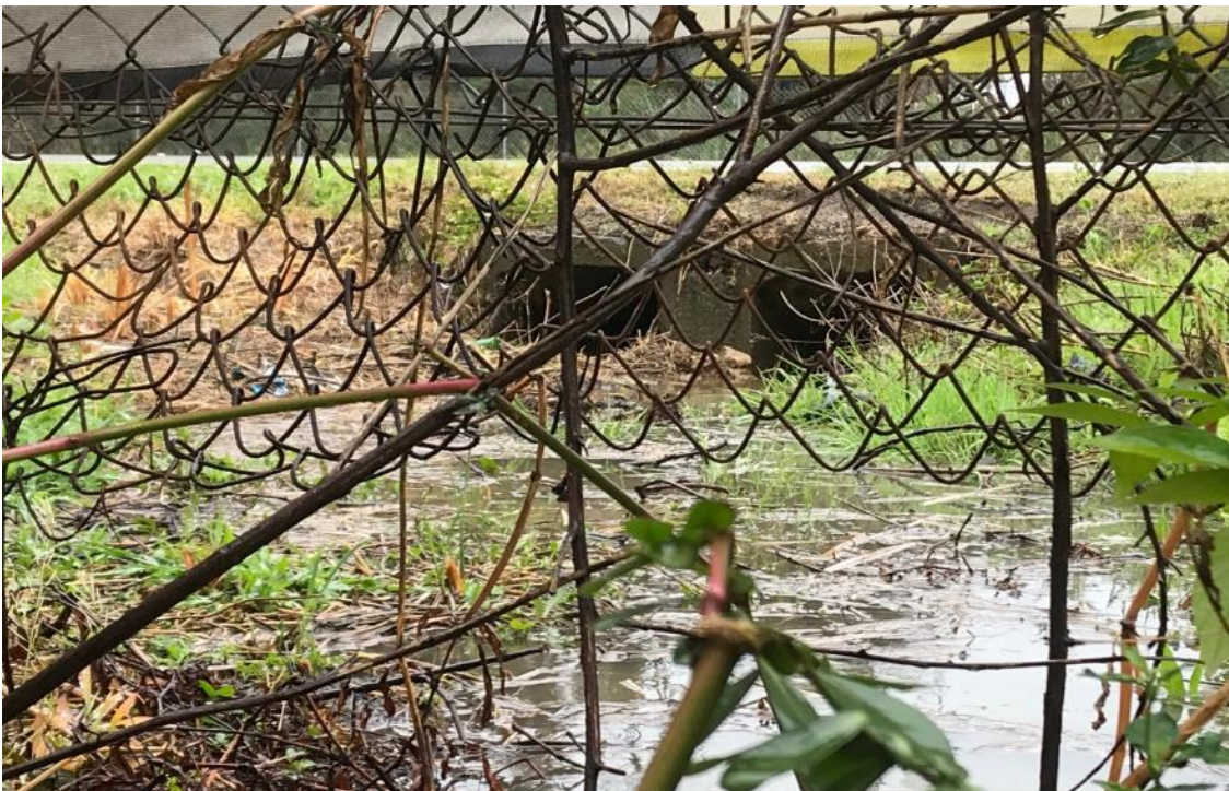
Photograph 4: Fence conditions at MPW site near existing Anzac creek culvert (18 Sep 2019)
