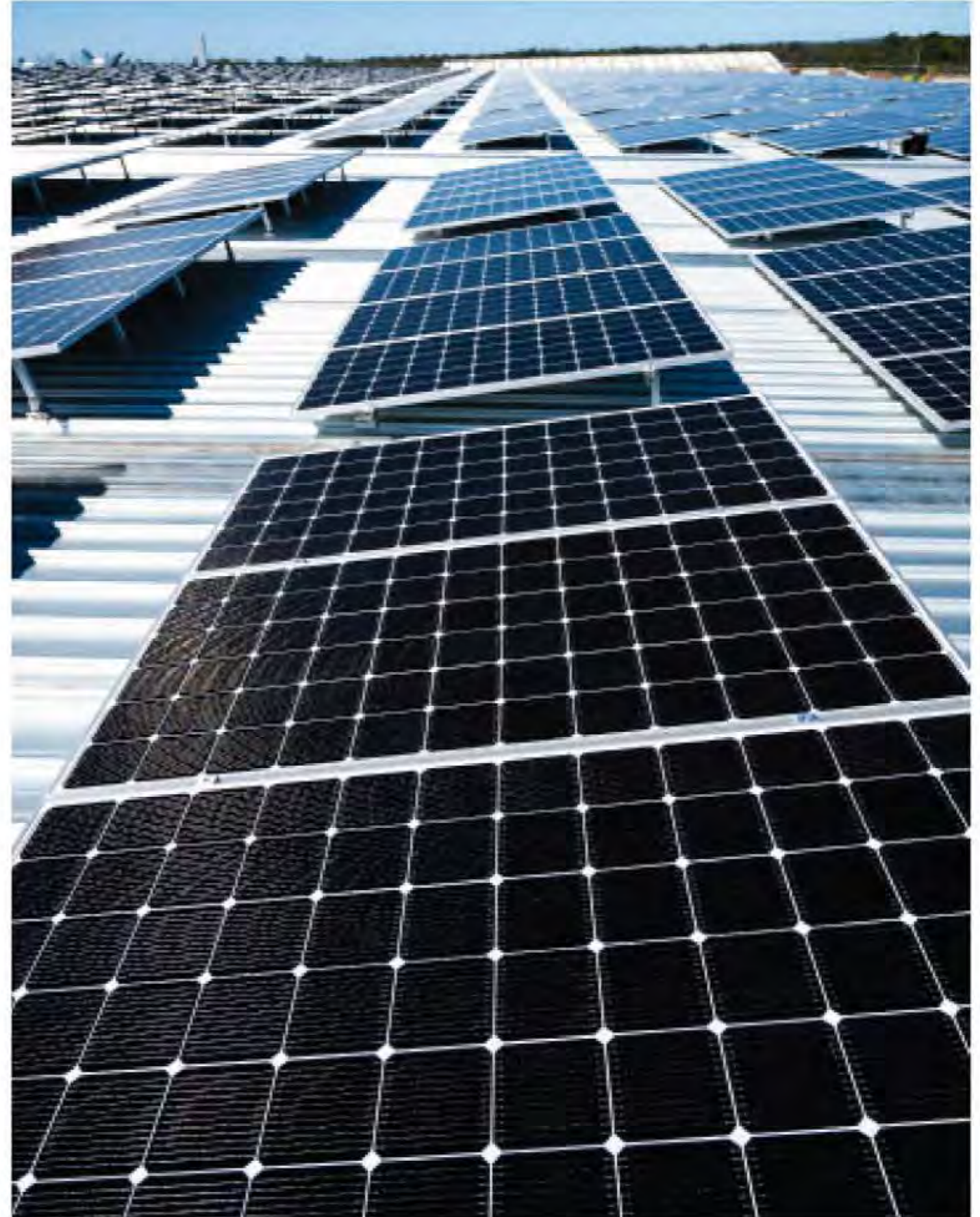
FIGURE 3.16 - Solar Panels installed at Development East Warehouse 1.
