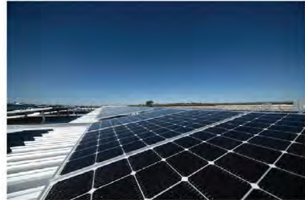
FIGURE 2.8 - Solar Panels installed at development East Warehouse 1. Alone, this installation generates 4,800MWh per year, or the equivalent of powering more than 7,300 homes.
