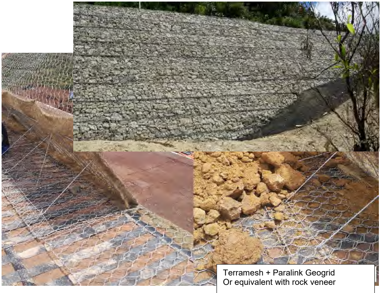
Figure O1: Typical details of Terramesh or equivalent facing with rock veneer
