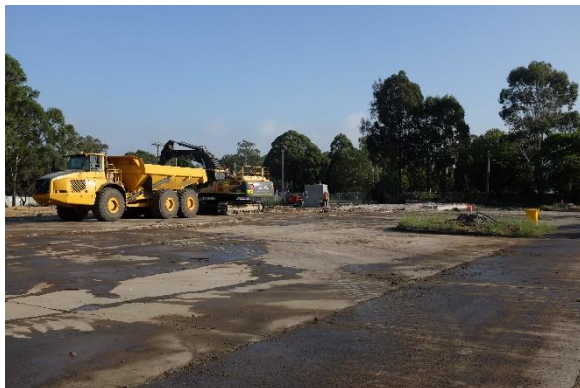
Figure 14. PAD W prior to concrete slab removal and archaeological investigations, view northwest.
