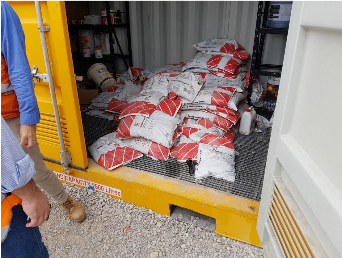
Plate 3: Bunded chemical store
