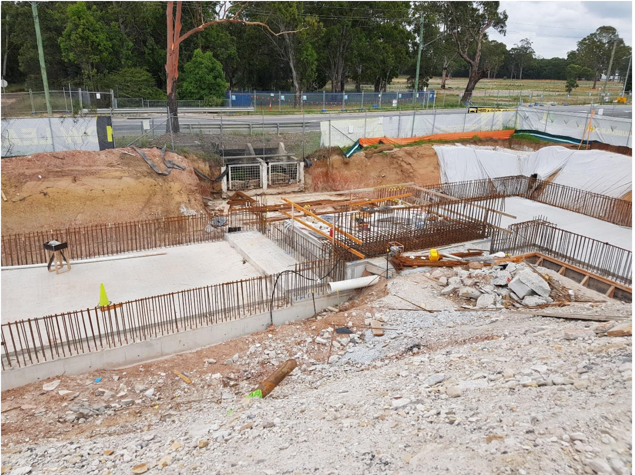
Plate 4: Outlet C (rear of photo) protected with sandbags from runoff from adjacent excavation and concrete works.
