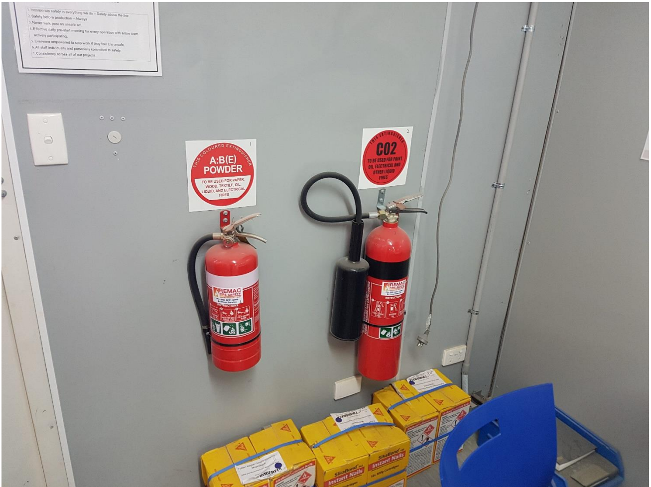
Plate 5: Fire extinguishers within Fulton Hogan site office
