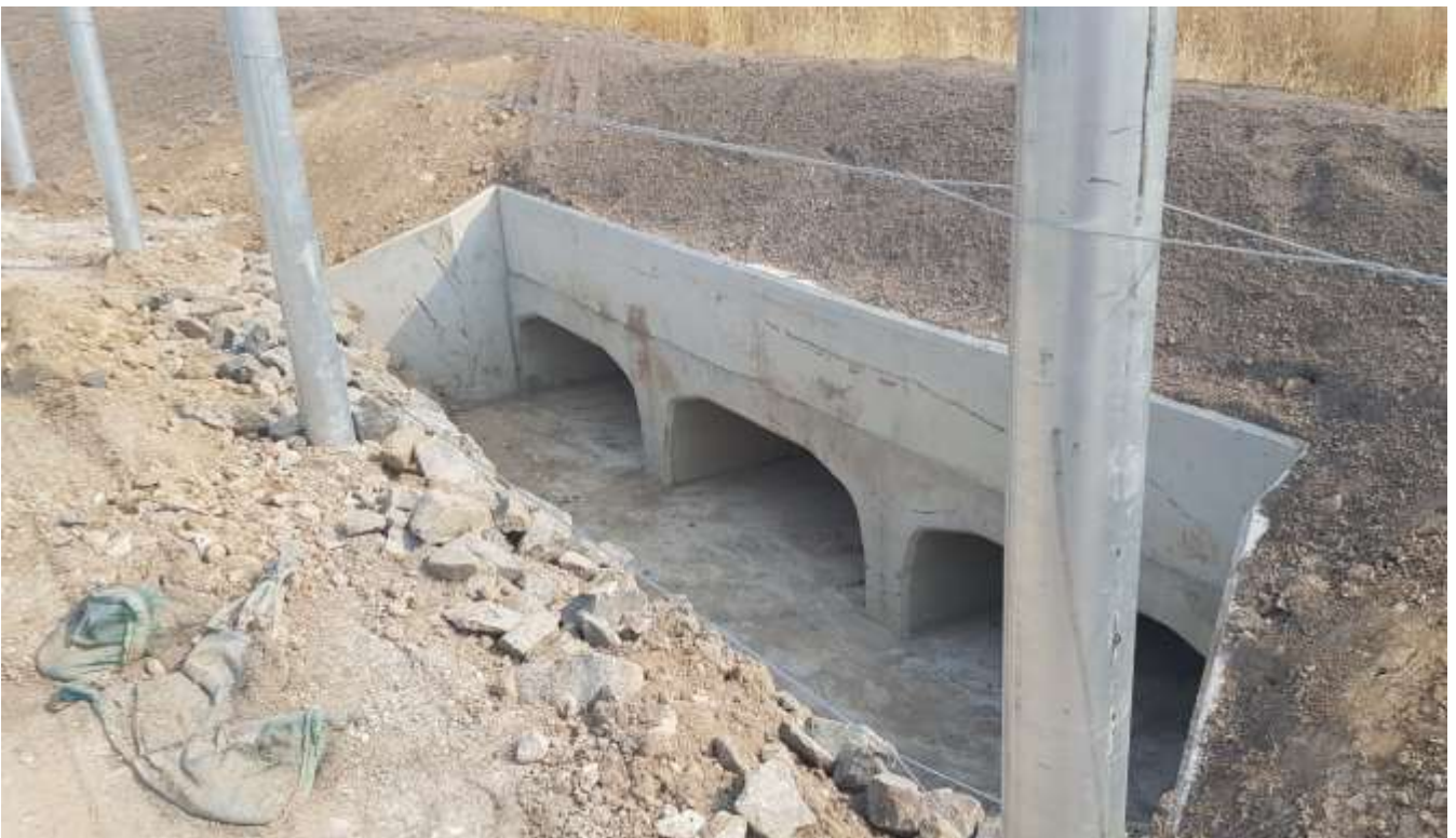
Figure 3: Stormwater culverts for drainage under the rail line.
