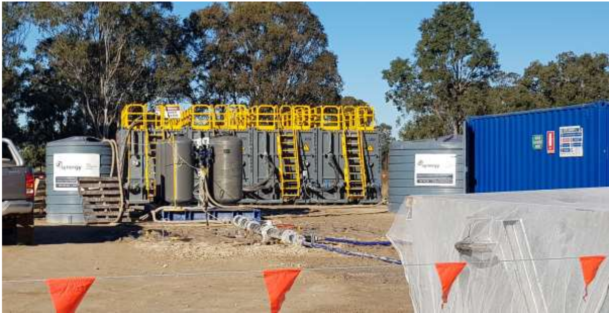
Photo 4: PFAS impacted water treatment plant
