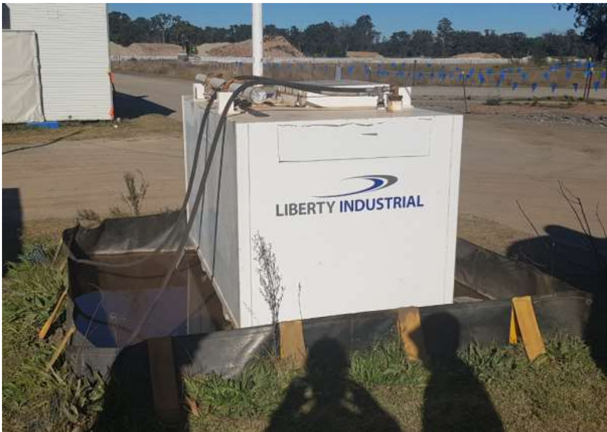
Photo 9: Bunded fuel storage
