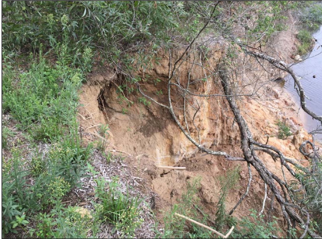
Figure 5 Existing 750mm outlet scouring (on the east bank of the Georges River)
