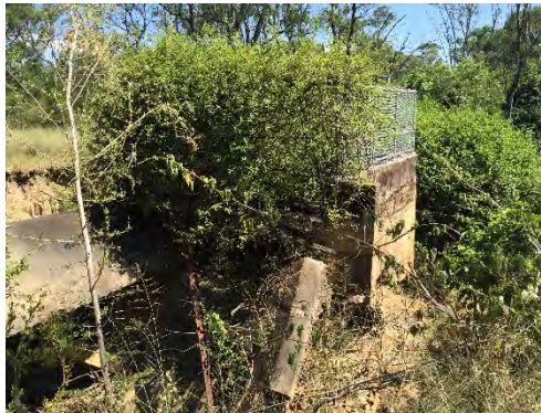
Existing damaged/collapsed drainage structure
