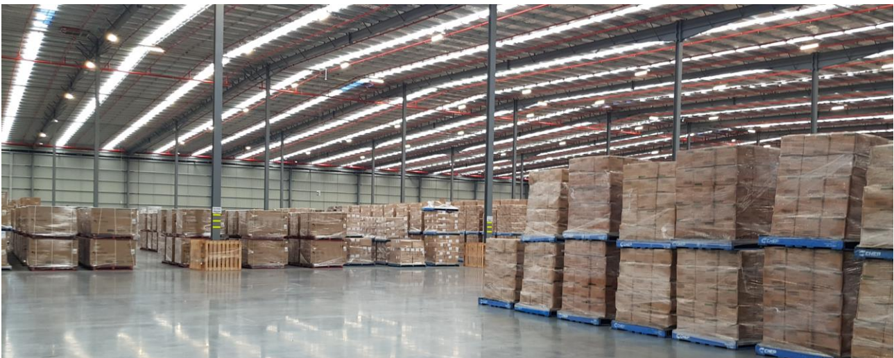
Photo 11: Passive and LED lighting design within warehousing.
