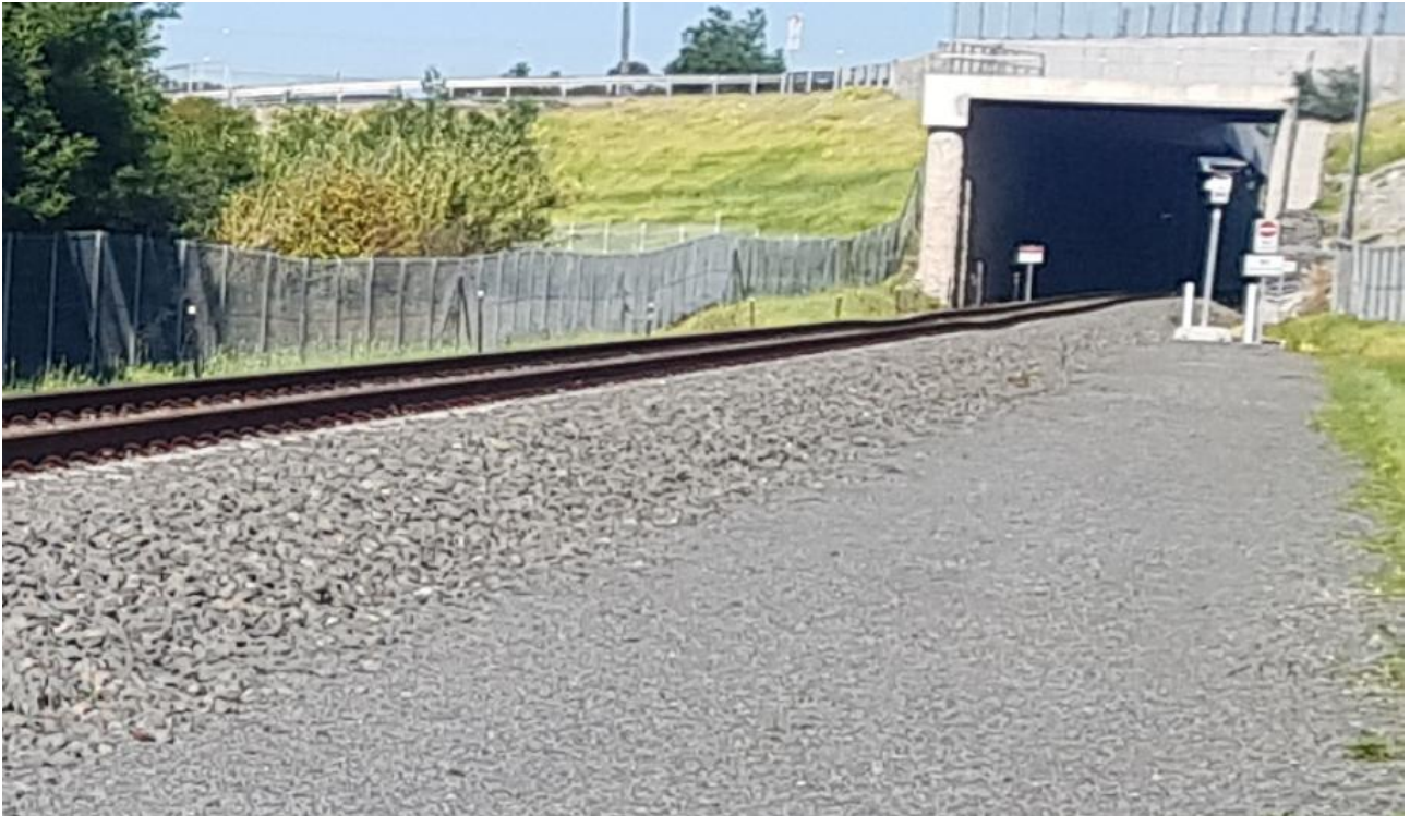
Photo 6: Rail Link buckling between IMEX Terminal and the Moorebank Avenue underpass.
