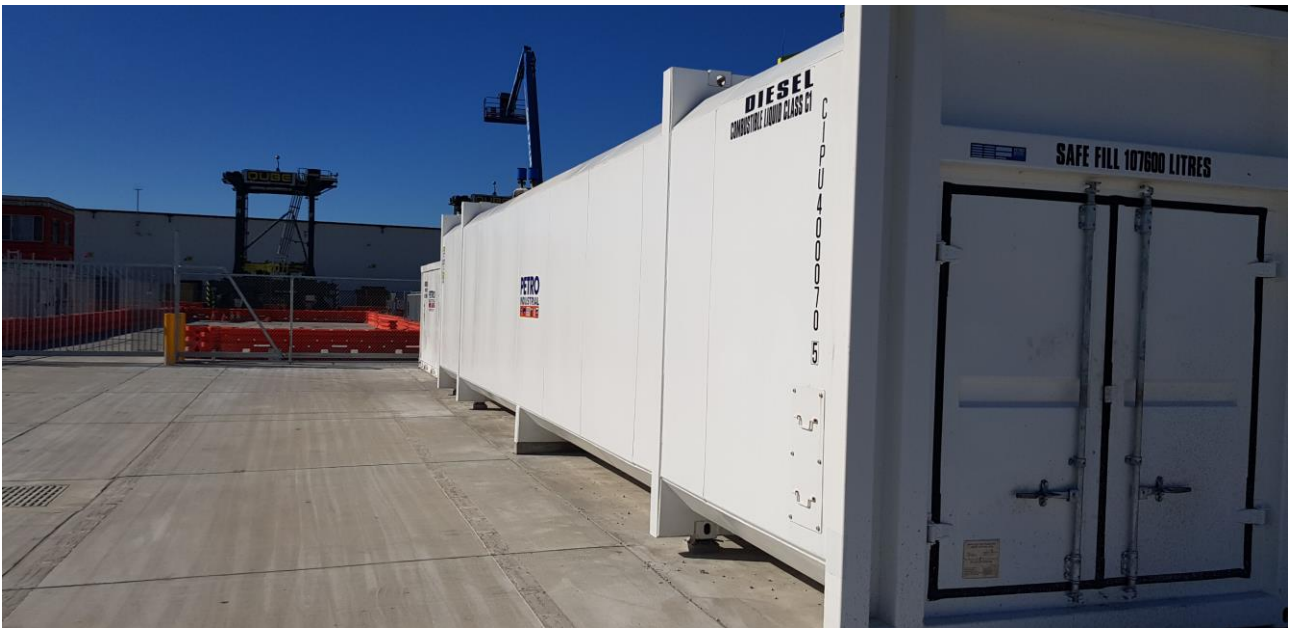
Photo 1: Bulk diesel storage on the IMEX Terminal.
