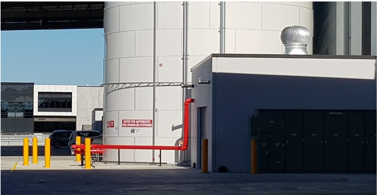
Photo 12: Firewater bulk storage for warehousing.
