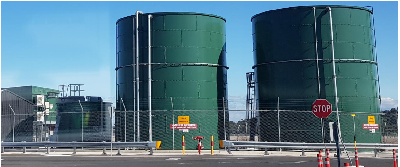
Photo 14: Firewater bulk storage for IMEX Terminal.
