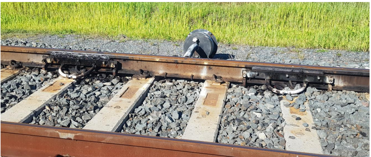
Photo 7: Rail Link lubrication.
