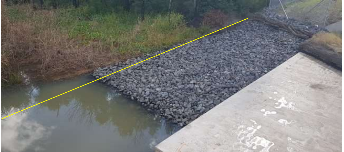
Photo 9: Anzac Creek 20 metre boundary breach (line shows approx. target alignment)
