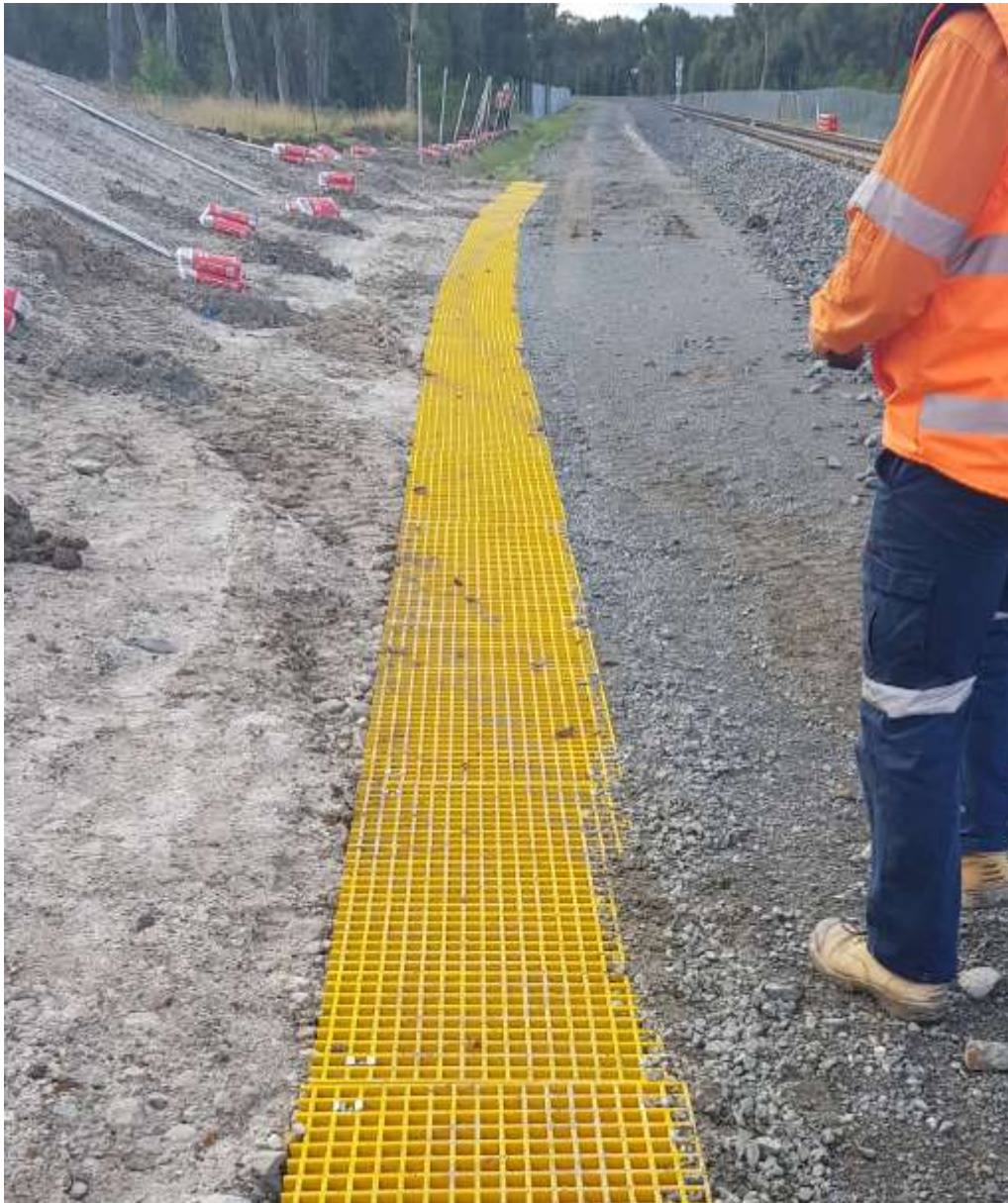
Photo 8: Operational drainage and fencing being installed in rail corridor adjacent to Bootlands
