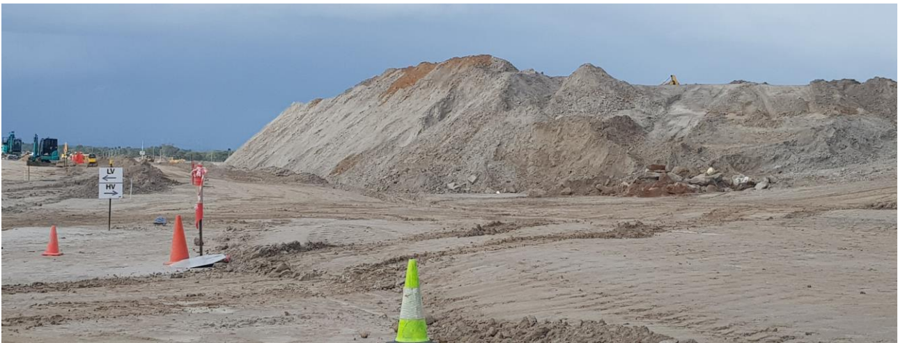
Photo 2: Example of stockpile not in compliance with CoC B43
