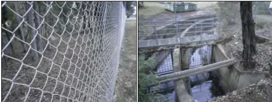
Photos show the concrete trapezoid within the site and the approach to the pipes crossing under Moorebank Avenue.
