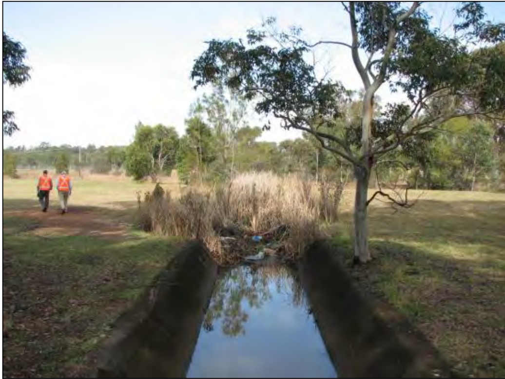
Photo shows concrete trapezoidal channel leading into heavily vegetated open channel which then drains to existing outlet on south-eastern corner
