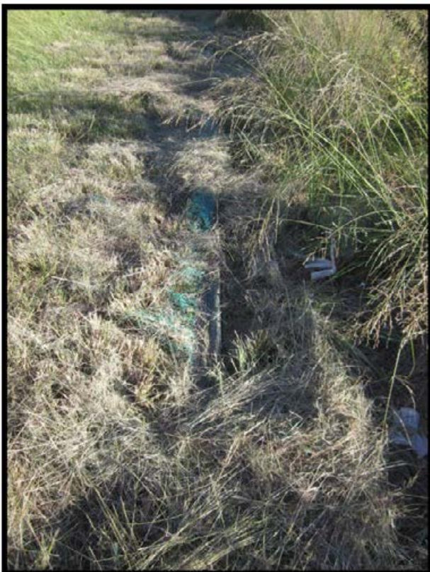
Photograph 6: Geotextile/silt fence identified along the central footpath in the central area of the site.
